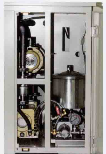
ES301+Vacuum Pumping Unit
